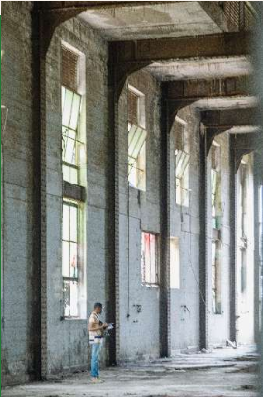
(Above) Image of interior of Ijora Power Station, 2024, Olájidé Ayeni, Team NowNow
